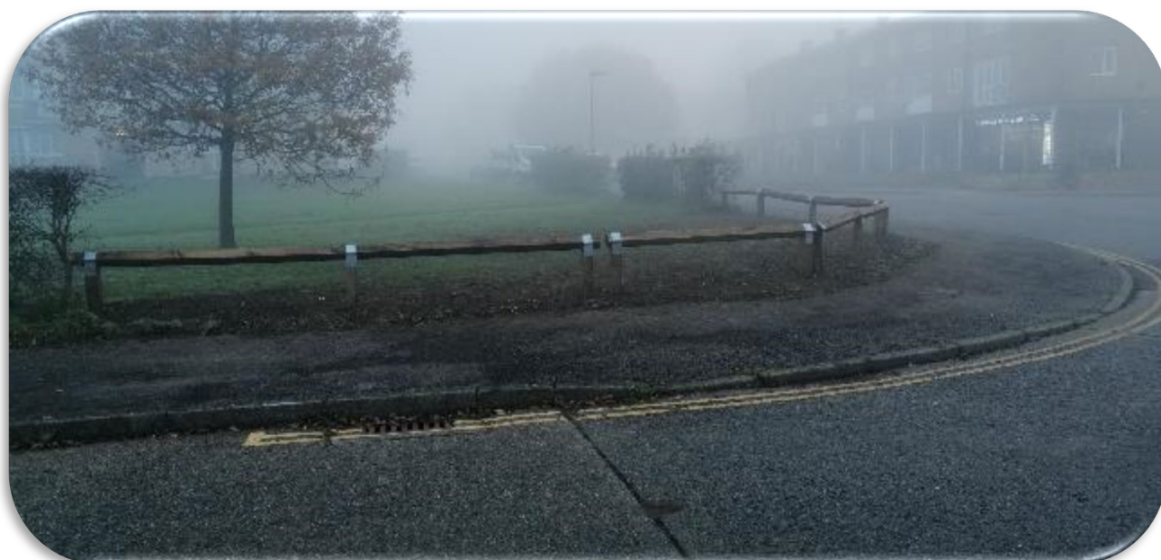
Figure 9: NW124 – Installation of knee-high timber rail barrier at Junction of Preston Lane and Marbles Way, Tadworth
