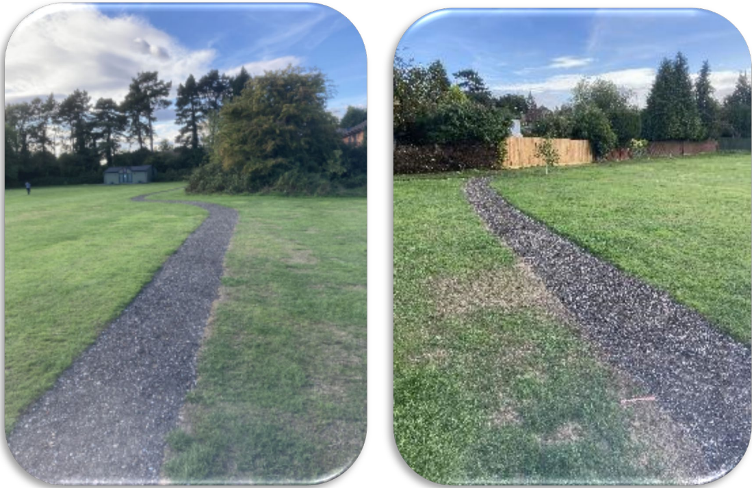
Figure 3: NW81 - The installation of an all-weather country path at Garton Recreation Ground, Garratts Lane, Banstead
