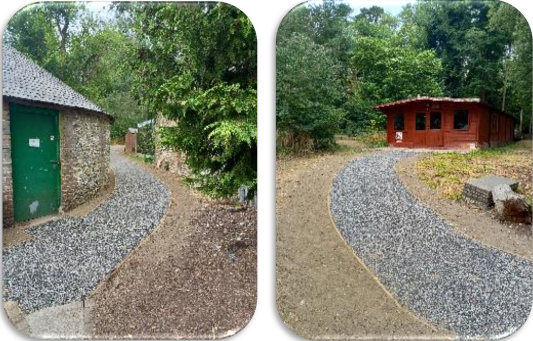
Figure 4: NW107 - The surfacing of informal paths to and through Park Farm Scout Camp Site with a permeable surface to improve accessibility.
