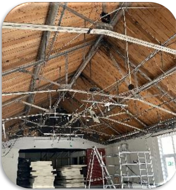
Figure 10: NE71 – To fund the replacement and improvement of the roof insulation at Kingswood Village Hall, Waterhouse Lane, Kingswood, Surrey
