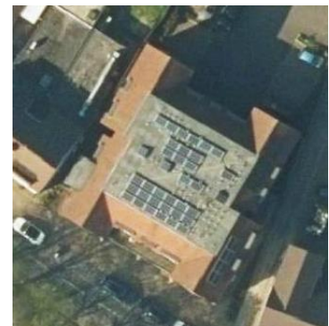
Figure 93: Many panels are being hidden within crown roof schemes in the borough. Image source: Google maps
