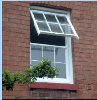
Figure 88: Mock sashes are unacceptable and disruptive to the building form.
