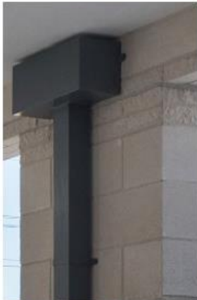
Dark grey aluminium rainwater pipes
