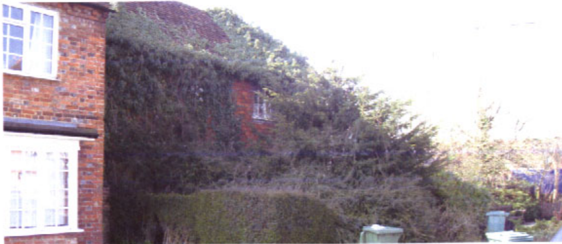
The overgrown state of this cottage will result in the long term witha repairs notice if it results in the structural deterioration of the cottage.
