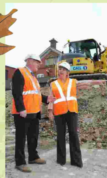
Photo: Paul Trevett (Facilities Manager, Southern Railway) and Cllr Kay Hammond (Surrey County Council) discussing progress at the station redevelopment site
